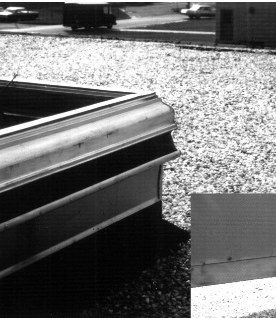
Installed CMAB (Curb Mounted Aluminum Base) prior to placement of rooftop unit.
